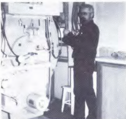
Emile Paradis, Plant Manager checking boilers. 1989.
