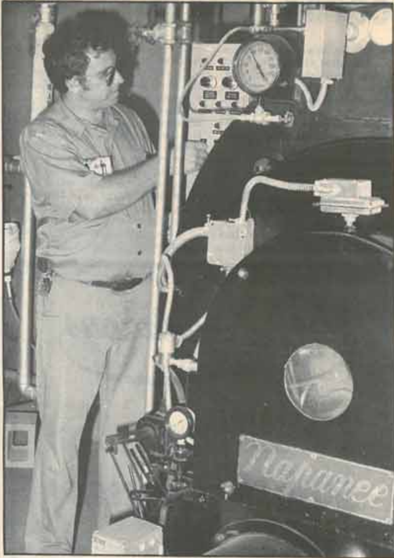
HIGH-PRESSURE STEAM BOILERS at St. Peter's Hospital are the responsibility of Lorne Pfeifer, director of the plant operations department.
