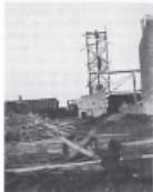
Hoist in place. Construction of St. Joseph's Hospital in progress at right. 1906.
