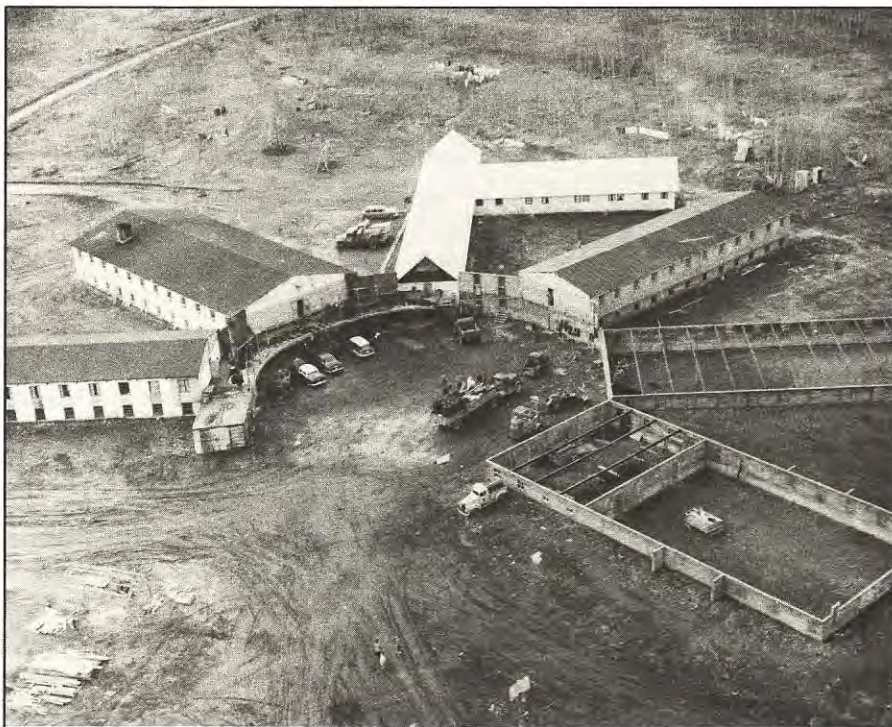
Copper Valley School under construction, as of 1958. The sisters' quarters were in the T-shaped building, the section stretching to the right. (SPA) (Photo credit: Copper Valley School, Public Relations Dept.)
