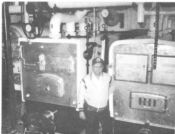
Brother E. Morin, Chief Engineer in the present boiler room. (boilers were converted to oil firing in 1961)
