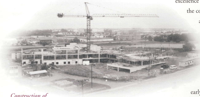
Construction of the new St. Joseph's Health Centre from Westmount Road, fall 2001.
